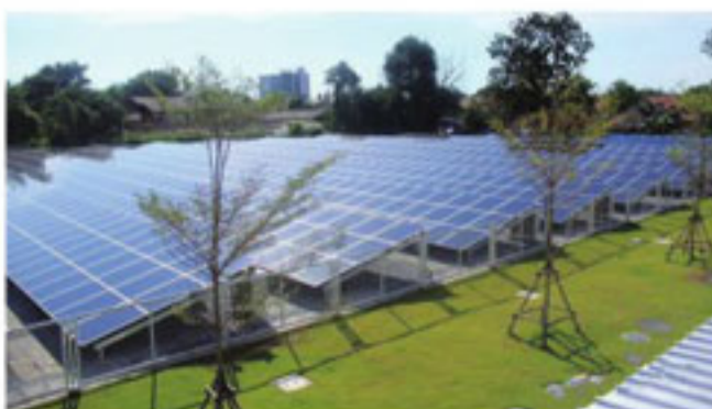
Farm Solar Generation System
