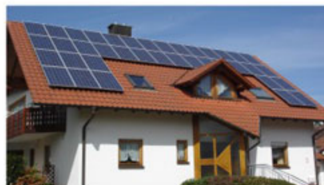
Off-grid Home Solar System
