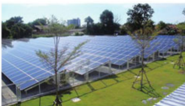
Farm Solar Generation System
