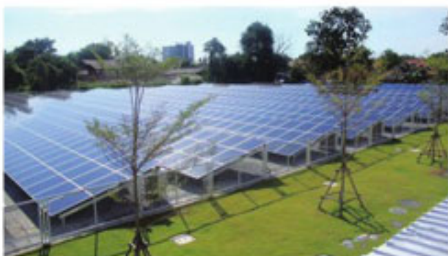
Farm Solar Generation System
