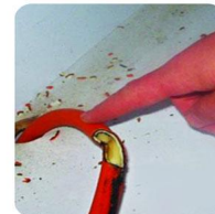
Pipe breaking cause gas leakage
