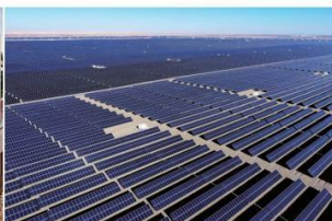
Surface power station
