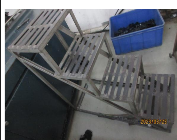
NC 7.17 No handrail for ladder
