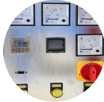
Clear operation control panel
