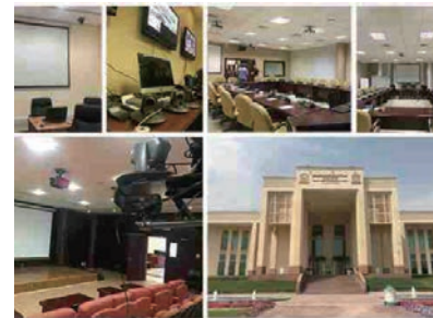
Lecturer Tracking Cameras Installed at UNESCO RCEP, UAE
