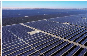
Surface power station
